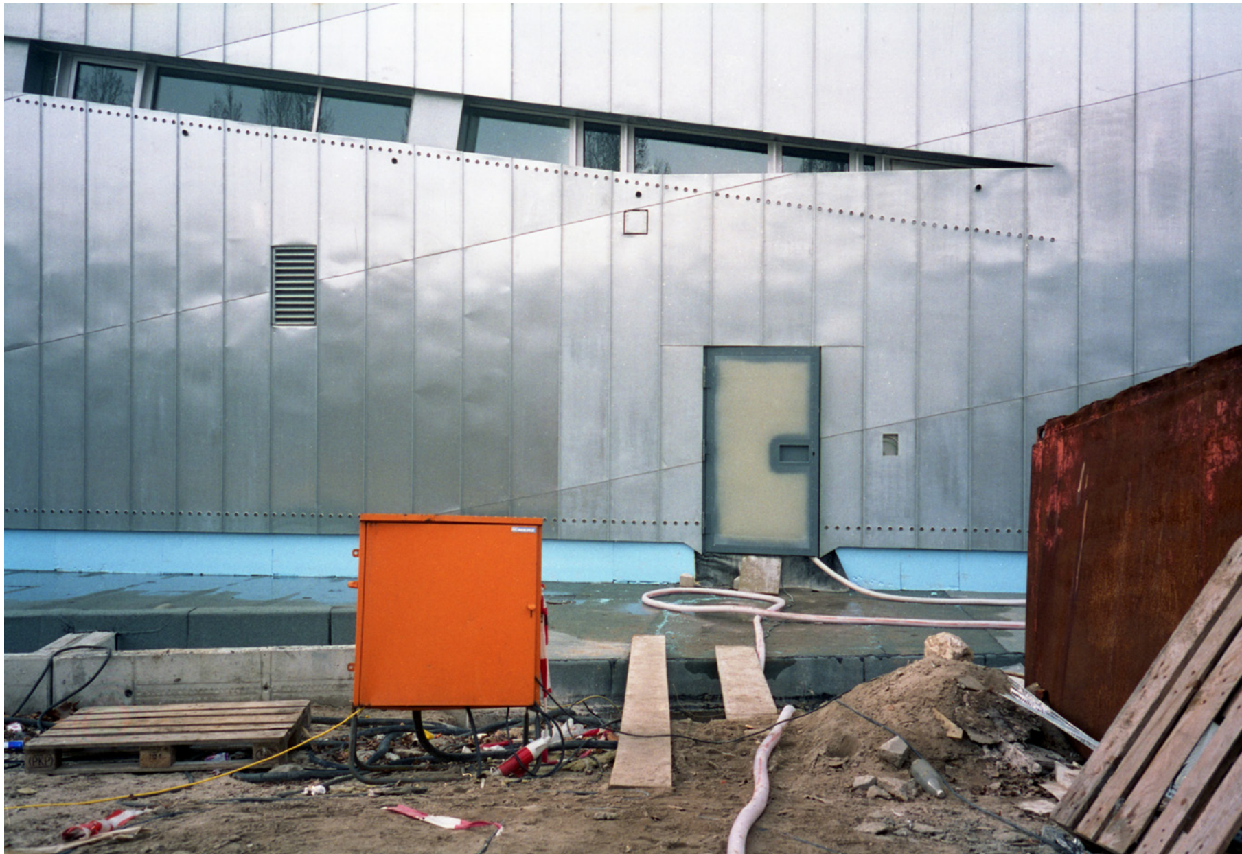
Daniel Libeskind, Jewish Museum under construction, Berlin, Germany, 1997, aus: Observation Is a Constant That Underlies All Approaches , Lars Müller Publishers, 2023, S. 206, © Phyllis Lambert
