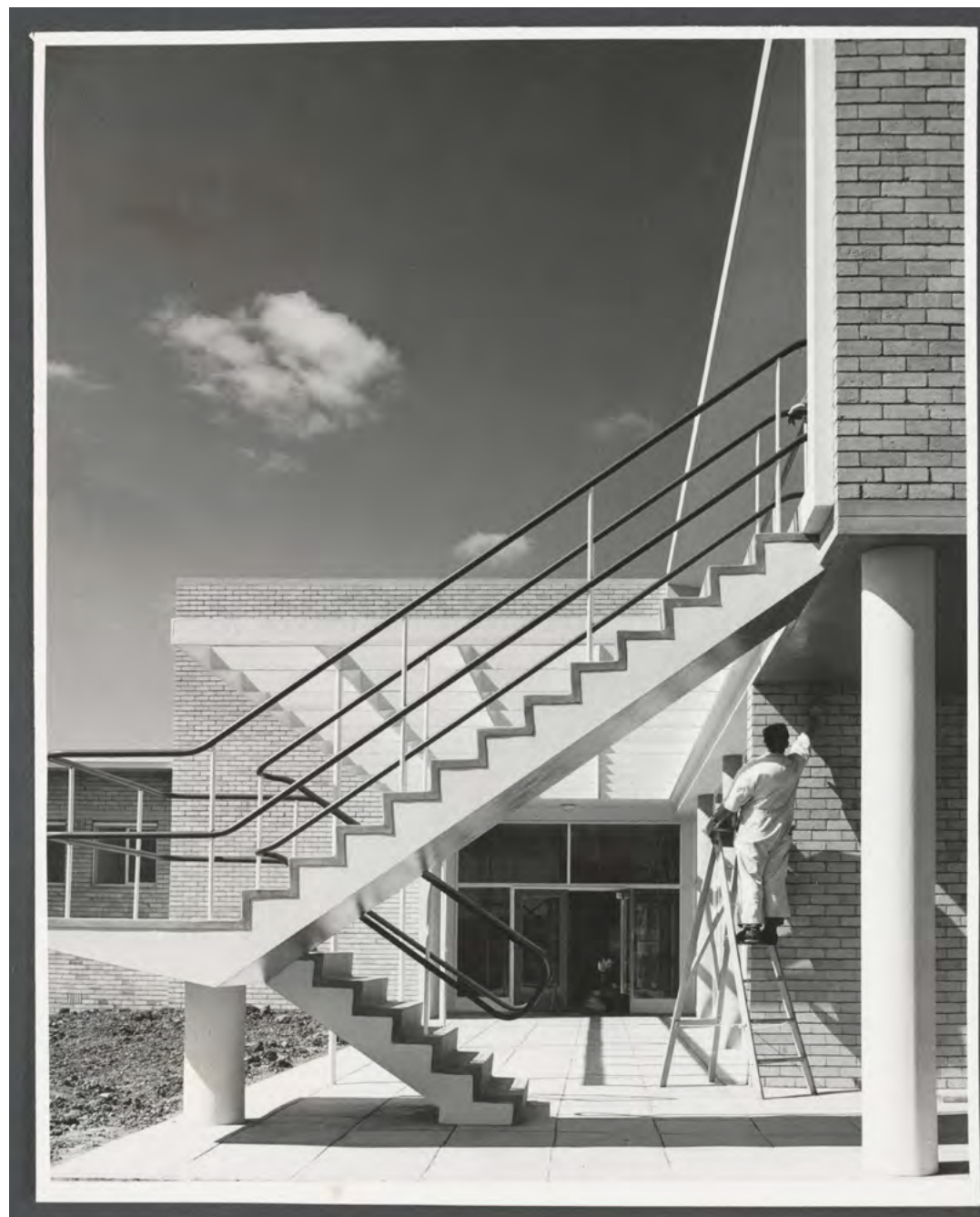
Workmen putting the finishing touches to rear of amenities block Foto: Helmut Newton, 1951-54
